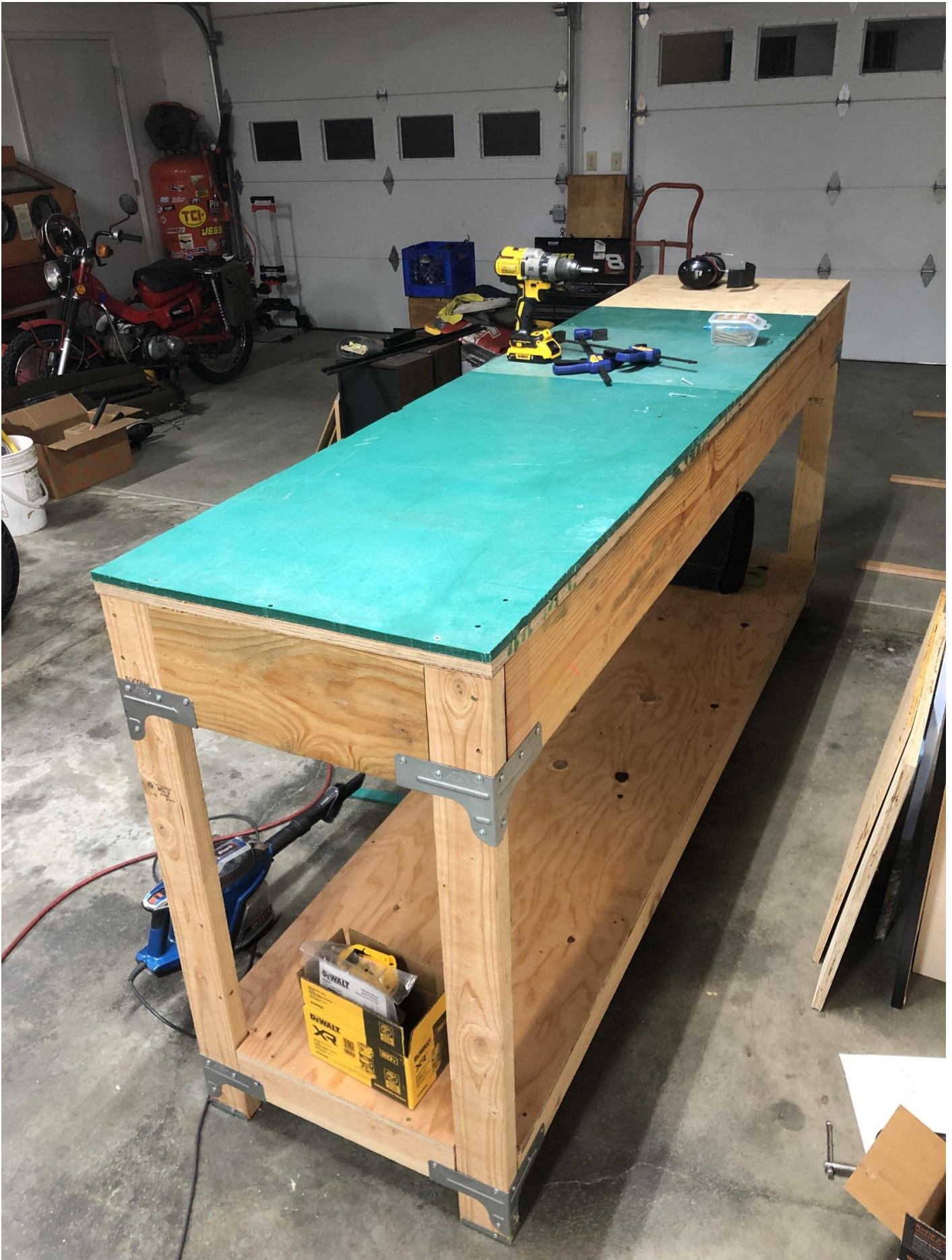
Built an 8ft long workbench. Used 2x4 and 2x8 lumber with an Simpson Strong-Tie WBSK workbench kit. Top and bottom shelves are 3/4 CDX plywood. Used pocket holes on the two end
